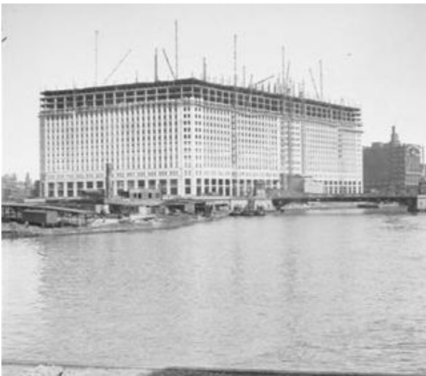
The Merchandise Mart under construction, seen from the Lake Street Bridge in 1929.
